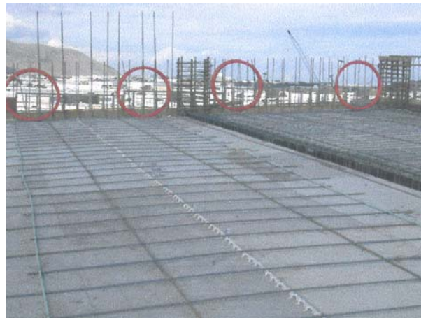
FIGURE 3b-2 Construction of a One-Way System, Where Bars are More Uniformly Spaced
